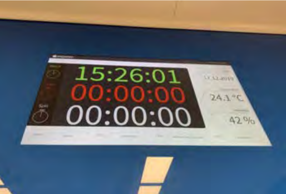
Digital clock connected to control panel
