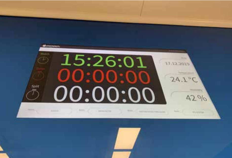
Digital clock connected to control panel
