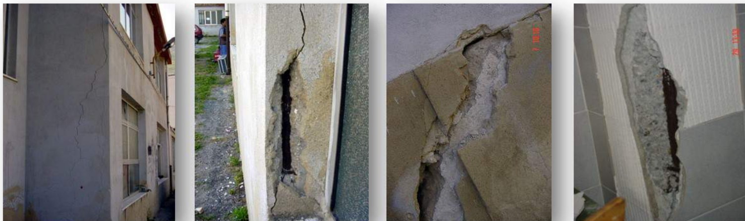
Survey of the crack pattern
