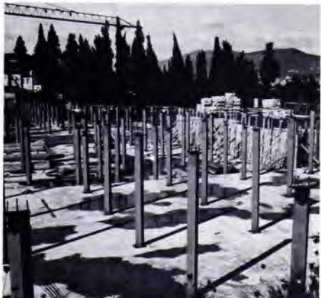
I pilastri in acciaio destinati a sostenere la copertura giardino scalinata in c.a. gettato in opera / Steel columns meant for the support of the stepped roof garden (the roof is built by in situ cast reinforced concrete)
