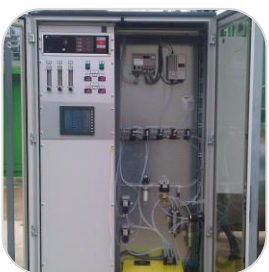
Analisi Biogas in campo
